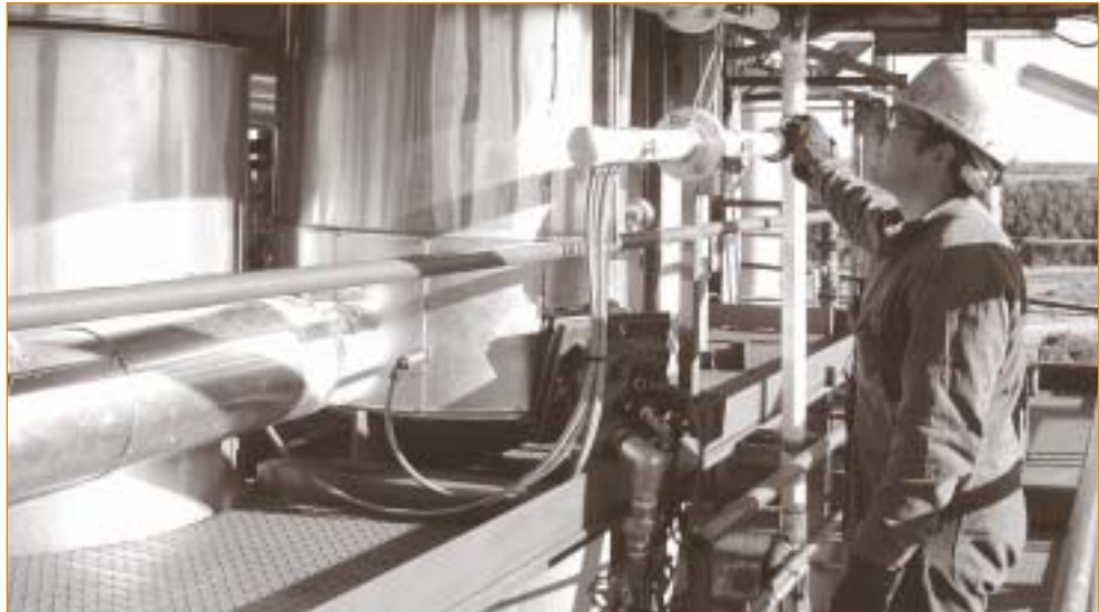
John Winter monitors the operation of the low temperature roaster and the efficiency of the after-burner
