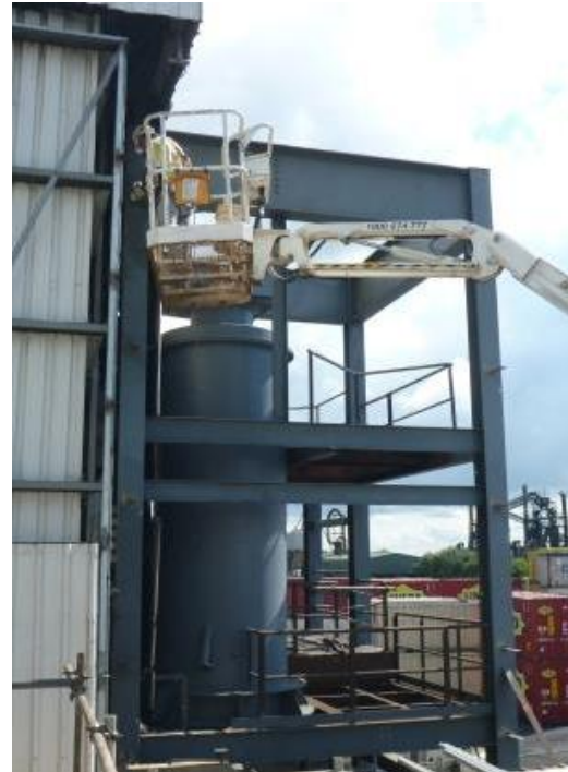
Installation of cleats on the refurbished process tower. The afterburner for the evaporation section has been installed
