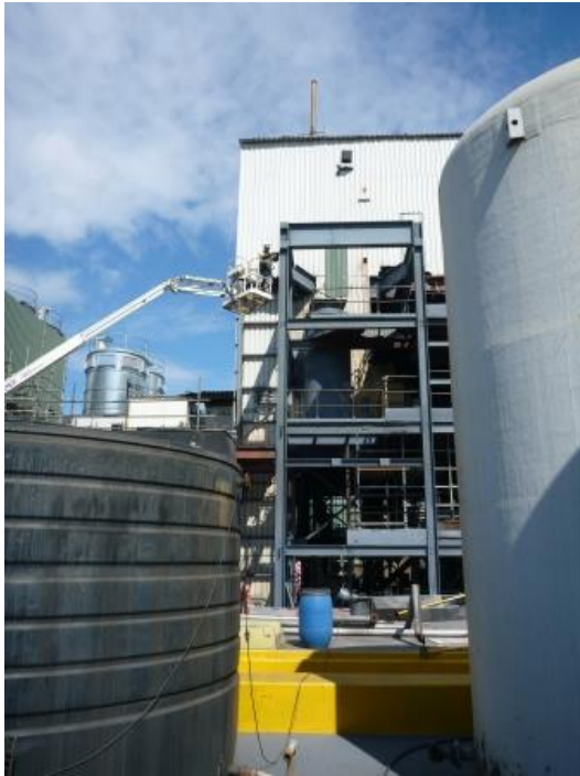
Refurbished process tower being prepared for the extension which will support the EARS acid regeneration and metallisation equipment
