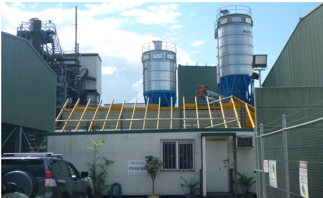
View of the Plant from the south showing the site office in the foreground, the new laboratory roof behind, the process tower to the left and the product silos and plant room in the background
