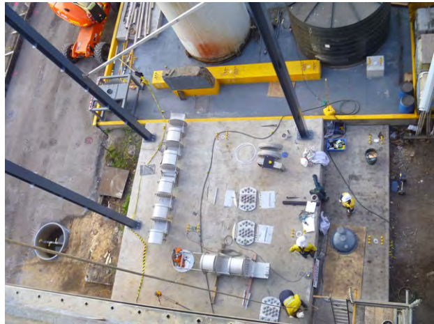
Erection of the steelwork for the northern extension to the process tower is underway. The EARS acid regeneration and iron reduction equipment will be installed in this section.
