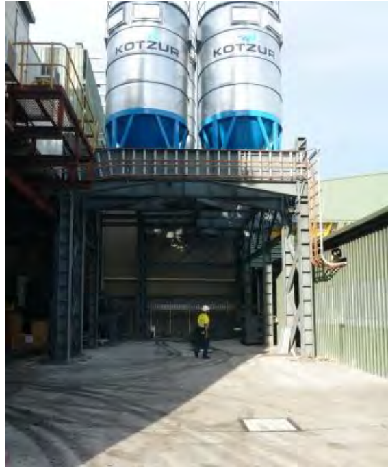
The reinforced concrete driveway for loading trucks with iron chips and char, as well as site drainage, is complete.
