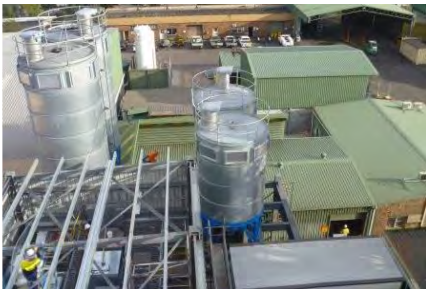
View of the southern end of the Plant, showing the plant room prior to the installation of the roof (lower left), iron and char product silos, workshop and laboratory (middle), mill scale shed (upper right) and bulk nitrogen and oxygen tanks next to the car park.
