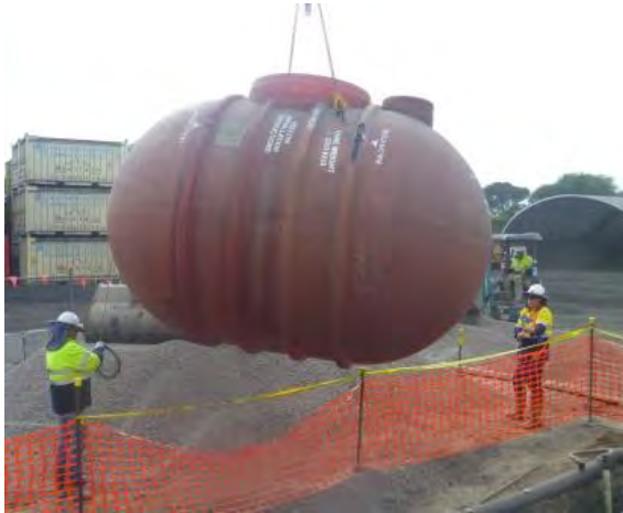
Installation of the sump tank beneath the tanker loading/unloading area is now complete.
