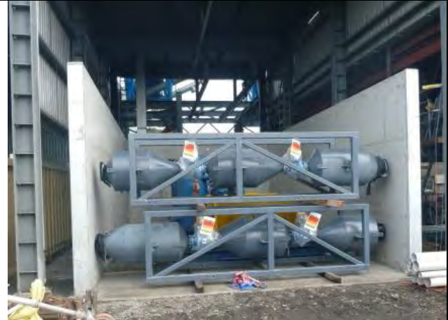
The completed iron briquette load-out bunker is being used to store lock hoppers for the coal delivery system.
