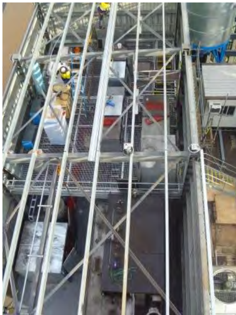
View of the plant room with mezzanine floor with blowers, compressors, waste heat boiler and hydraulic pumps in place.
