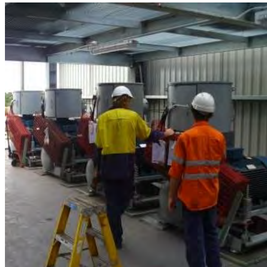
Electrical connection of the blowers on the lower floor of the plant room is underway.
