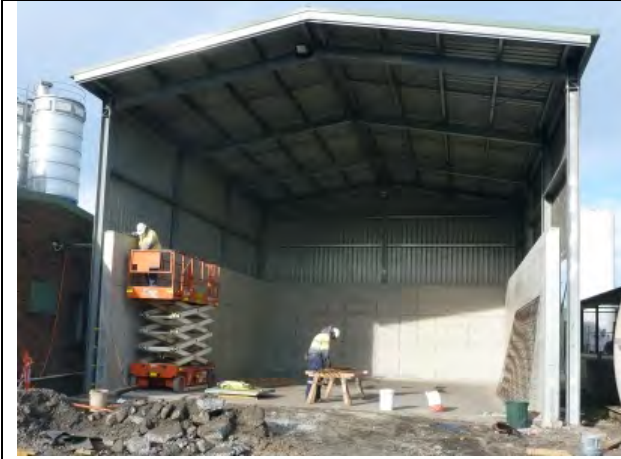
The bunker for bulk deliveries installed in the mill scale shed has a capacity of 800 tonnes.
