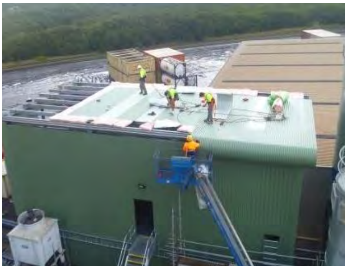
Installing the roof on the plant room. This houses the blowers, compressors, the waste heat boiler and the hydraulic pumps
