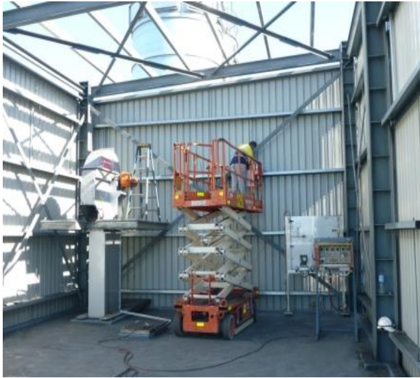
Installing brackets for the mezzanine floor in the plant room. The iron briquette bucket elevator is to the left and the oxygen panel to the right
