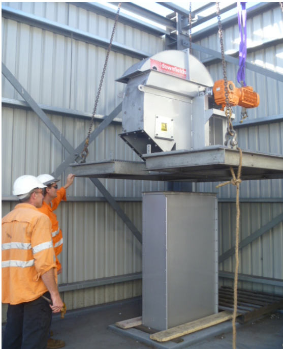
Installing the drive head of the bucket elevator used to transfer the briquetted iron product
