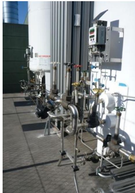
The bulk nitrogen and oxygen storage tanks are now connected to the Plant
