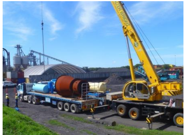
Delivery of the coal hopper, high pressure air and syngas receivers, and a fluid bed roaster for the iron reduction section
