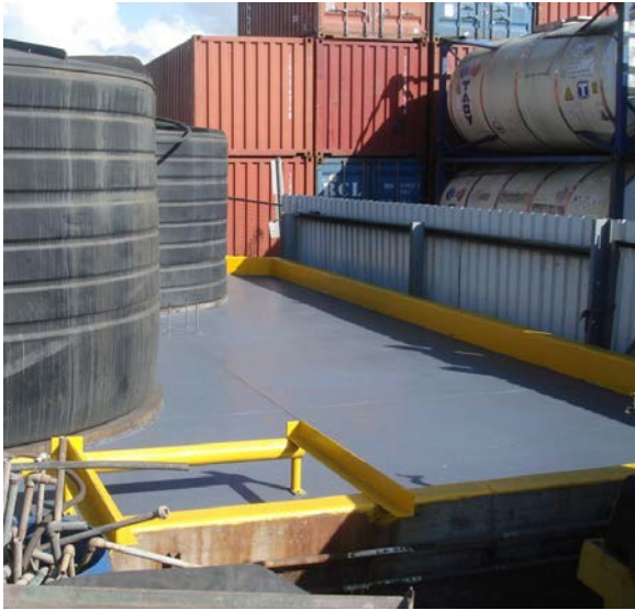
Tank farm bunded area with acid-proof epoxy sealant
