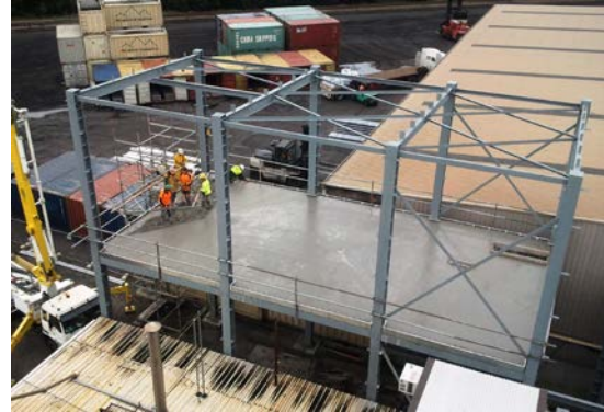
Above: Floor of elevated plant room
