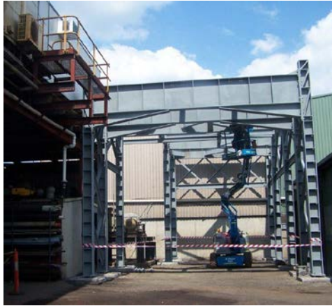
Structure for iron and char product silos and briquette binders
