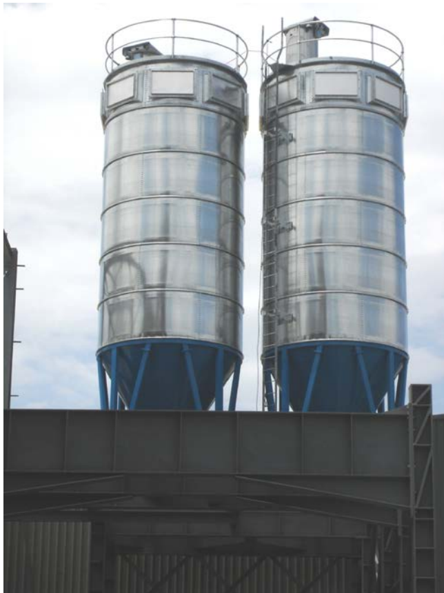
Each silo has a capacity of 37 m 3 and can hold 110 tonnes of product
