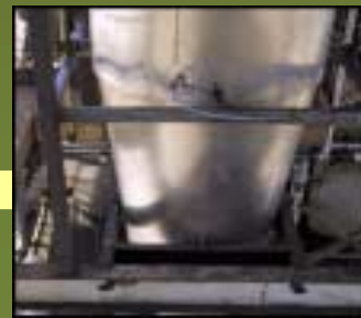
EARS acid regeneration plant
