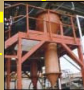
ERMS leach vessels
