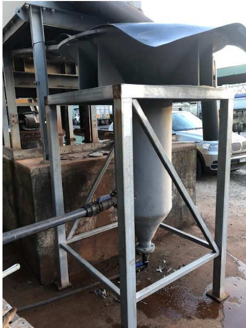
Fluidised furnace dust slurry feed tank
