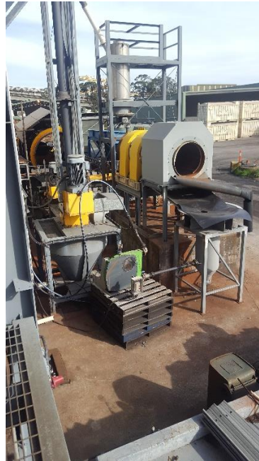
Dust slurry feed preparation area
